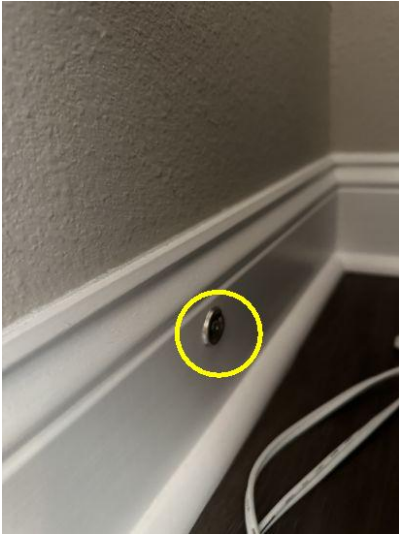
Center bedroom door stopper is broken.
