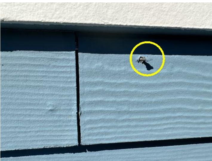
Cement siding (hardie board) has several nail pops; recommend re-nailing and sealing as needed.
