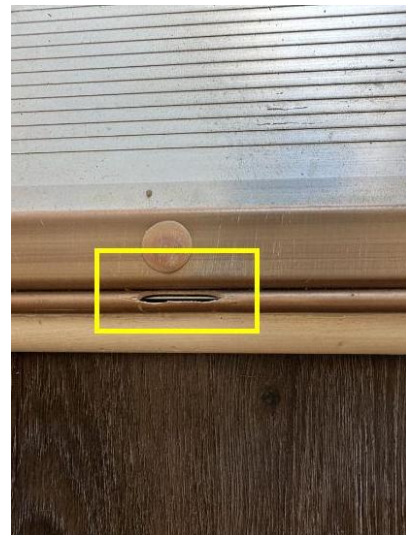
Small tear in the weather stripping along the bottom of the front door.
